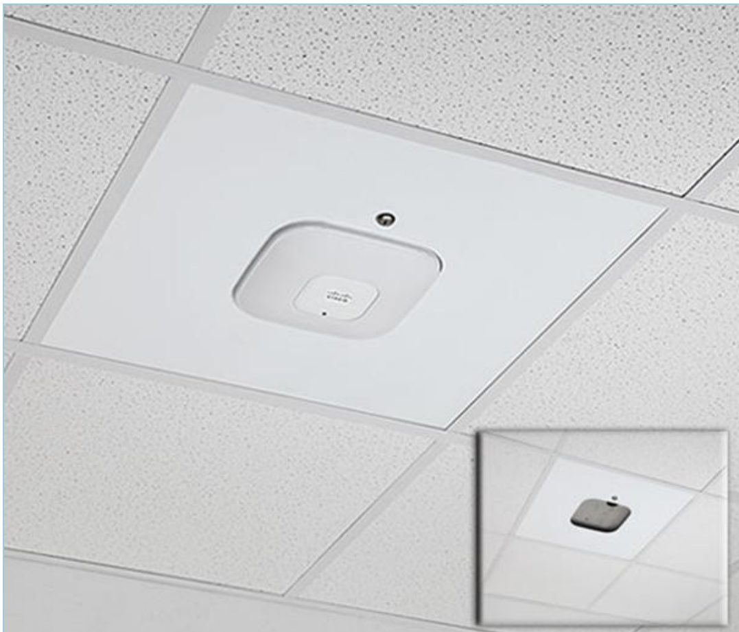
Figure 24: Oberon Metal Enclosure
